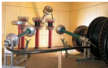
Figure 3 : Ultra Modern Hv Testing Lab
