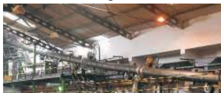
Figure 1: 6 Nos. CCV (DRY CURE) LINES
